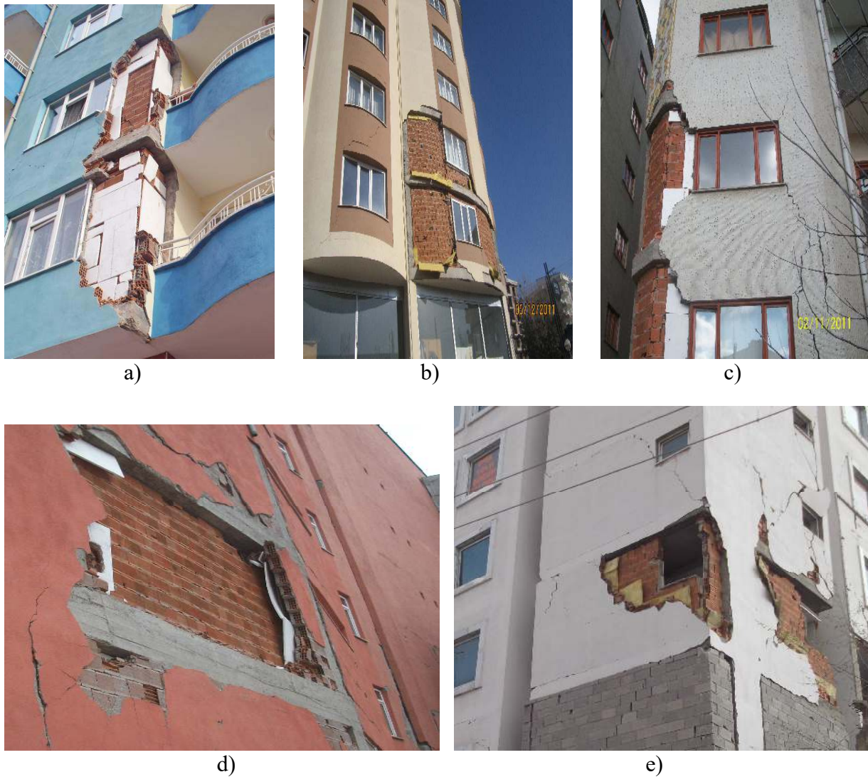
Figure 4. Failures of multi layers infill walls during the Van earthquakes
